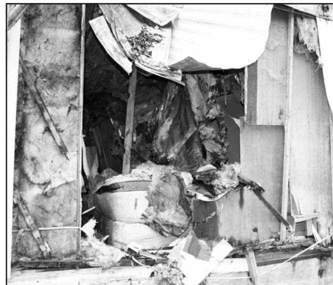
This is an interior view of the bedroom after the fallen tree was cut up and removed by a neighbor of the Hendersons. Photo by Shawn Jarrard
